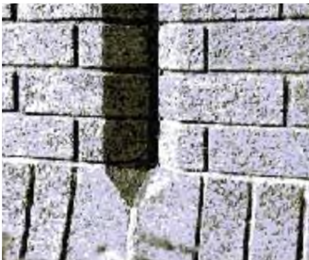
Photo 3 Accentuated Expansion Joint
